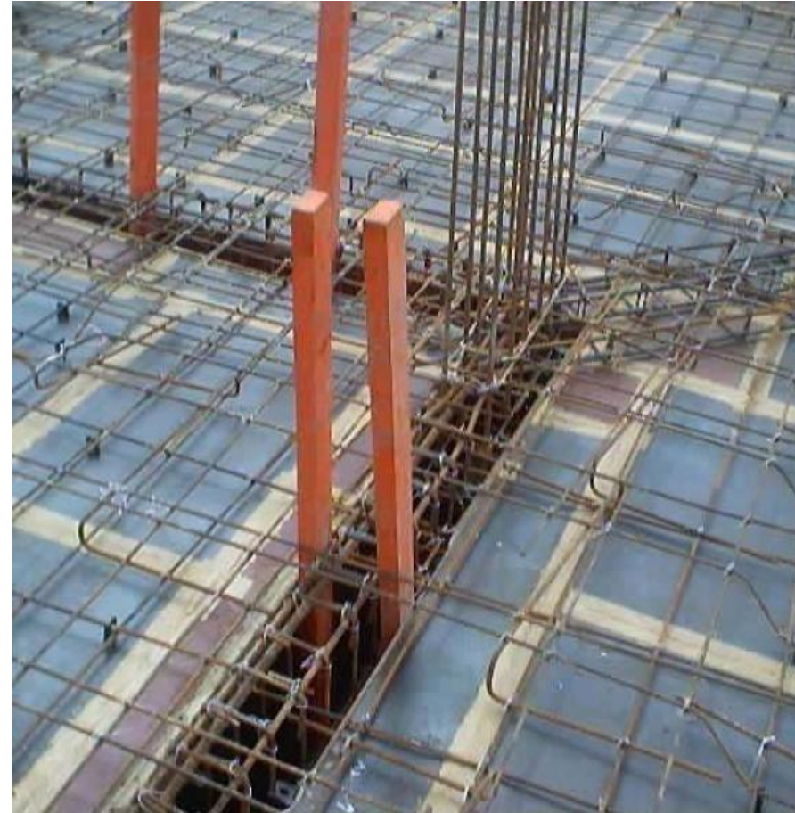
A wooden piece ("Kanda") instead of concrete cover for beam reinforcement
