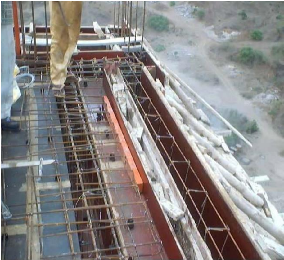
A wooden piece ("Kanda") instead of concrete cover at the chajjah / slab edge
