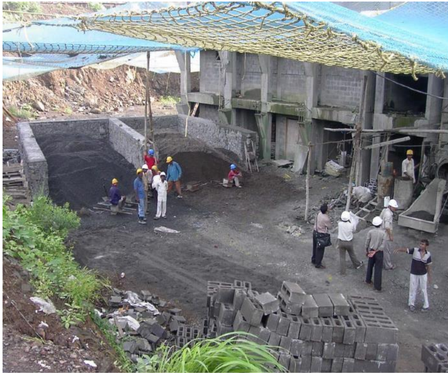
Site Batching Plant Permanent Cement go down and covered material storage
