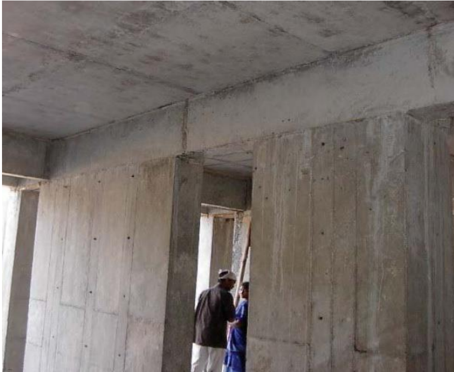
Quality of shuttering A pleasing look of Column - beam and slab beam junction
