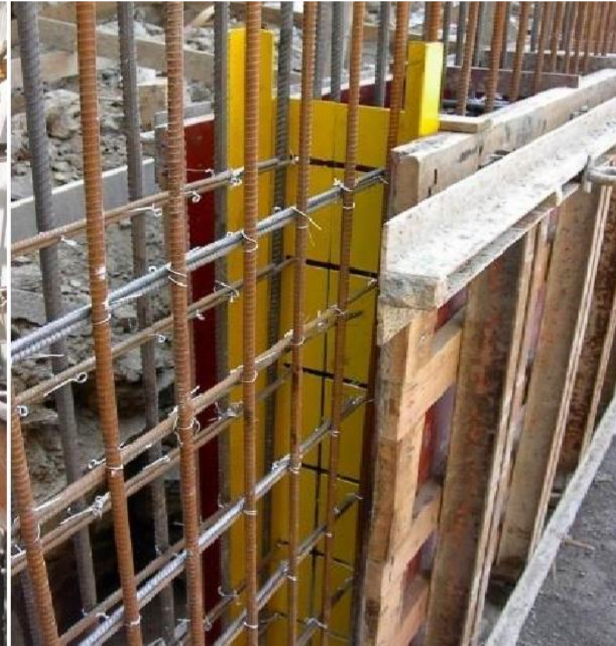
Vertical joint in the retaining and RCC parti wall. Joints left open for reinforcement to be sealed.
