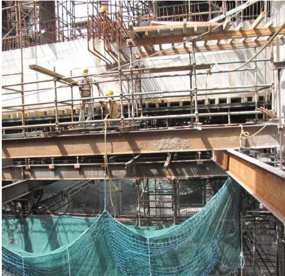
Steel platforms outside the building line to support multi storeyed staging and scaffolding
